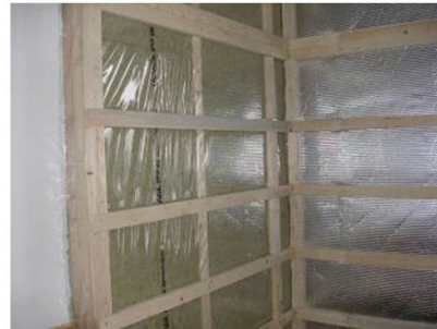
Fig. 2: Interior insulation of the log wall (left - option I; right - option II).
