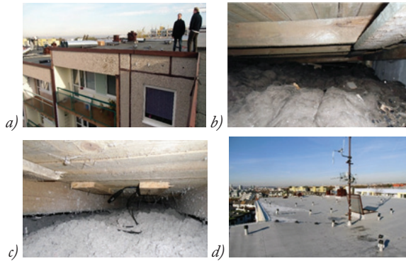
Fig. 7: Cold deck flat roof of a multi-story slab block residential building before and after retrofit. a) overall view, b) upper deck made up of assembled wooden elements and original mineral wool thermal insulation, c) additional cellulose thermal insulation, d) finished roof with additional roof vents.
