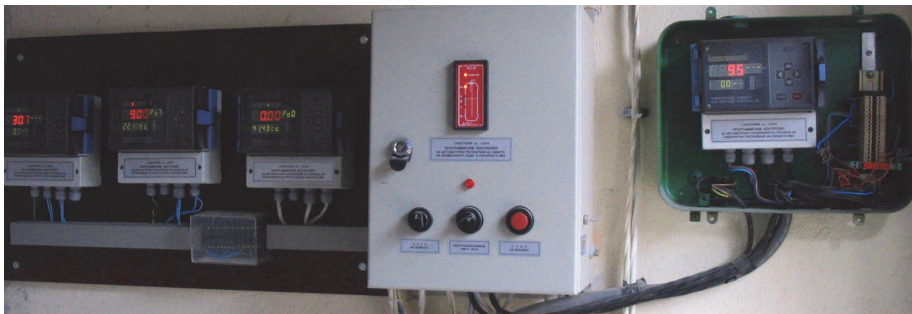
Fig. 8: Controllers for automatic computation and regulation of the steaming process of logs and prismatic wood materials (on the left and on the right) and for the leading away of the condensed water from the steaming equipment (center)
