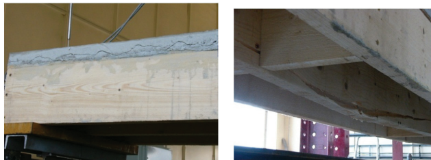
Fig. 6: Failure modes of the experimental timber-concrete composite beam.
