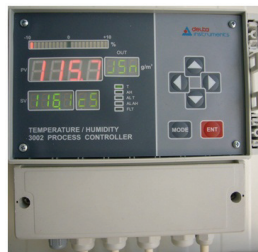
Fig. 8: Programmable controller for model predictive control of the thermal treatment processes of frozen and non-frozen wood materials.
