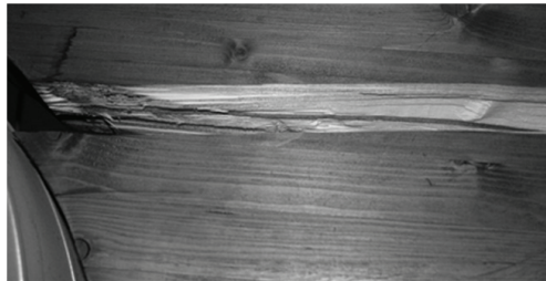
Fig. 6: Sever climate induced damage at the pit of the lamellas (unheated indoor environment).
