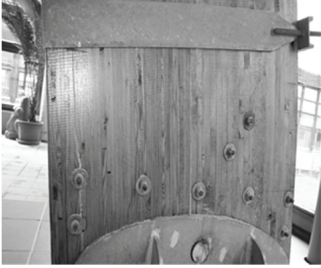
Fig. 3: Delamination of an indoor beam at the support; tied with metal brace (humid indoor environment).
