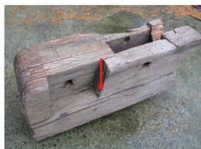
Fig. 2: The ending of roof construction element with short pieces of wood along the grain cut with grooves for other constructional elements (church in Boguszyce).
