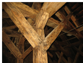
Fig. 1: Typical roof construction of a 16–18 th century church in Central Poland (arrow – shear strength; here: The church in Ceglów, 16 th century.
